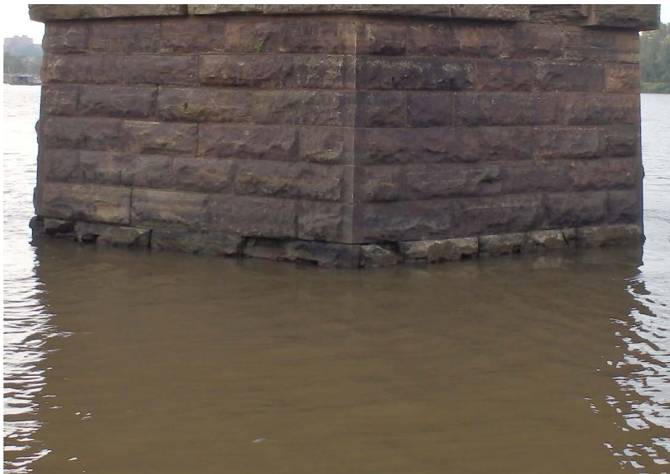
Photo 22 – Typical masonry stone loss and cracking surrounding the waterline
