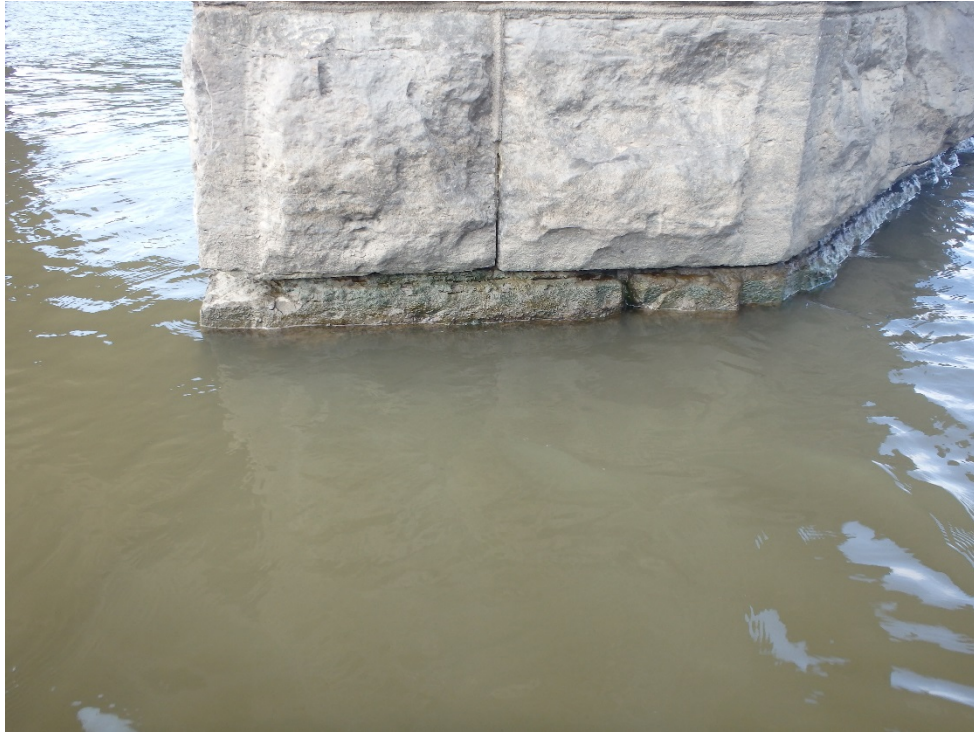
Photo 21 – Typical mortar joint loss within the freeze-thaw zone
